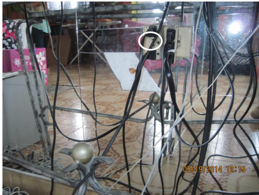
Photograph 10: No protective covers for electrical outlets, and exposed electrical cables and electrical cords in children's play area.
