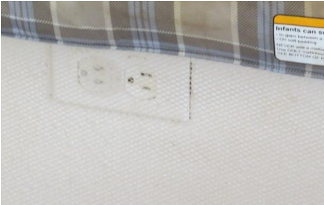
Photograph 5: An exposed electrical outlet was next to a crib.
