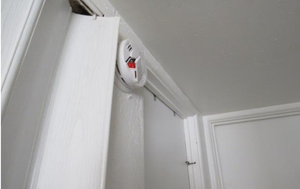
Photograph 7: The home's smoke detector was disconnected.
