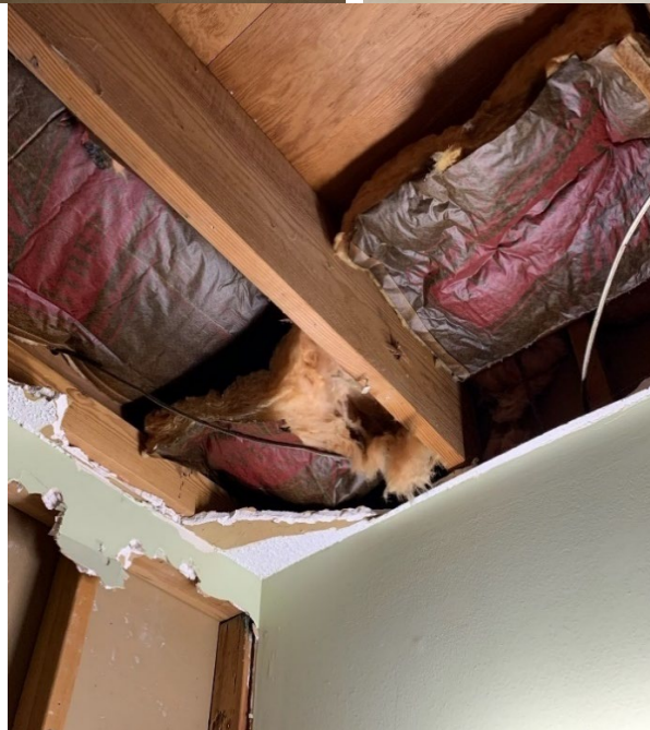
Photograph 1 (upper left): Opening in ceiling. Photograph 2 (upper right): Missing ceiling tile. Photograph 3 (bottom): Ceiling missing completely.
