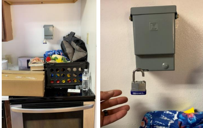
Photographs 7 (left): Stove, which is accessible to residents, covered in flammable items and therefore not properly maintained or inspected.
