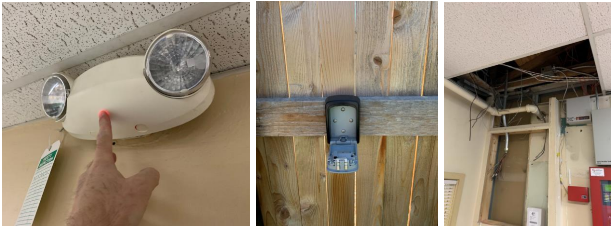
Photograph 4 (left): Non-functioning emergency light. Photograph 5 (center): Key, used to unlock gate in path of exit, missing from its lockbox. Photograph 6 (right): Hole in ceiling and wall at fire alarm control panel.
