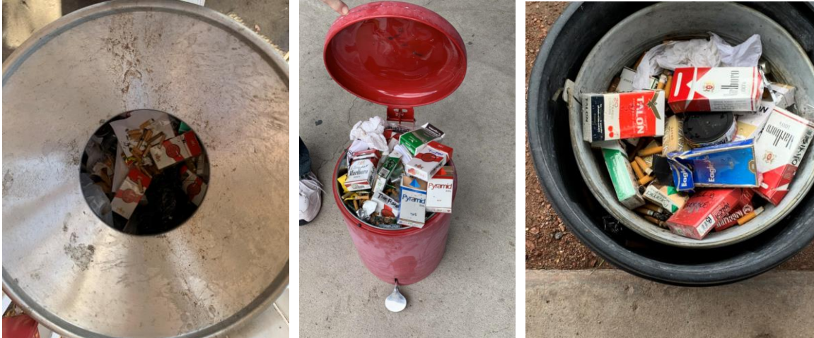
Photograph 14 (left): Improper disposal of smoking materials in trash container with combustible materials.
