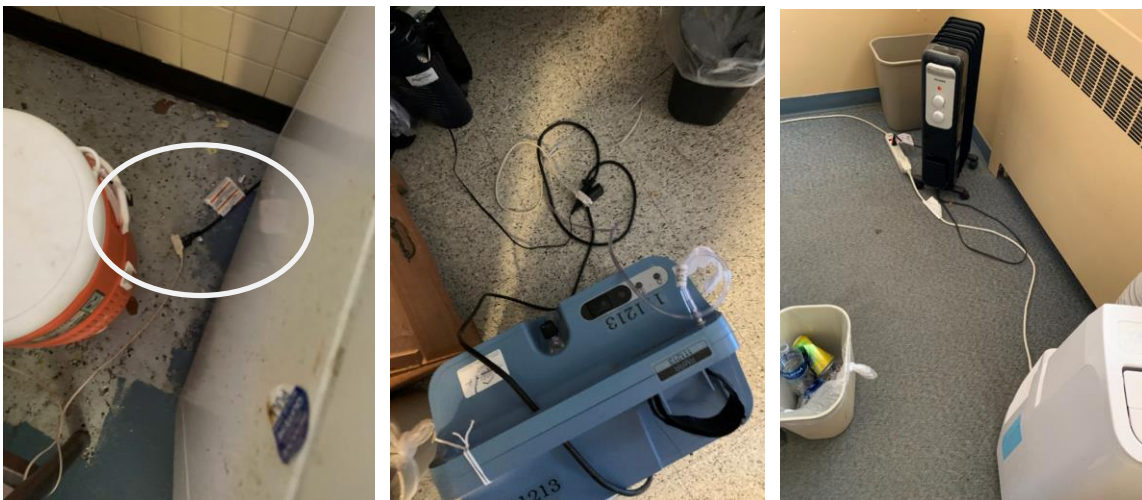
Photograph 17 (left): Kitchen refrigerator plugged into extension cord.
