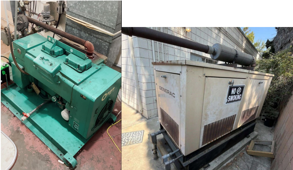
Photograph 1 (left): Generator manufactured in 1972. Photograph 2 (right): Generator manufactured in 1980.
