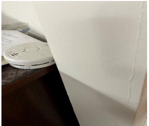
Photograph 4: Smoke Detector inoperable and not mounted
