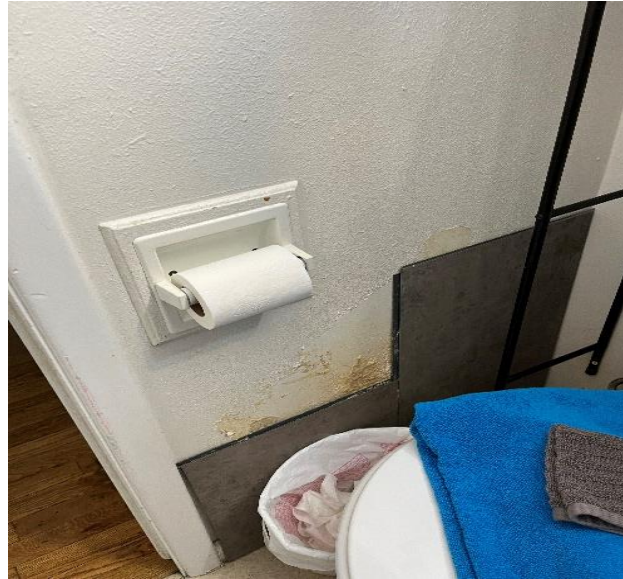
Photograph 10: Bathroom wall in disrepair with peeling paint
