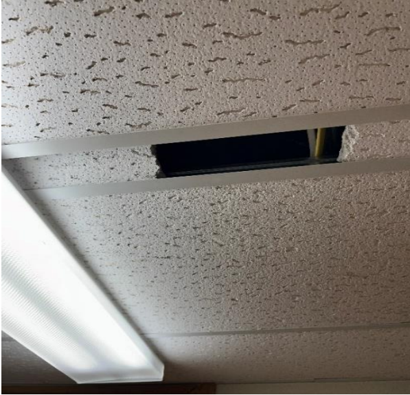
Photograph 15: Broken, missing ceiling tiles in basement
