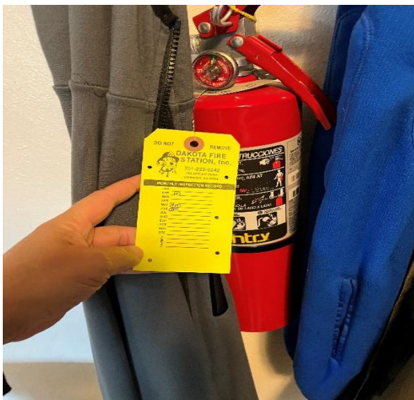
Photograph 19: Fire extinguisher mounted but covered behind sweatshirts and inconsistent monthly inspections (last inspection was June 2024) (Photo taken Aug. 28, 2024)
