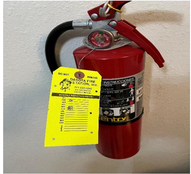
Photograph 12: Fire extinguisher with inconsistent monthly inspections (last inspection was June 2024) (Photo taken Aug. 28, 2024)
