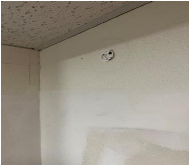
Photograph 3: Smoke Detector removed from wall
