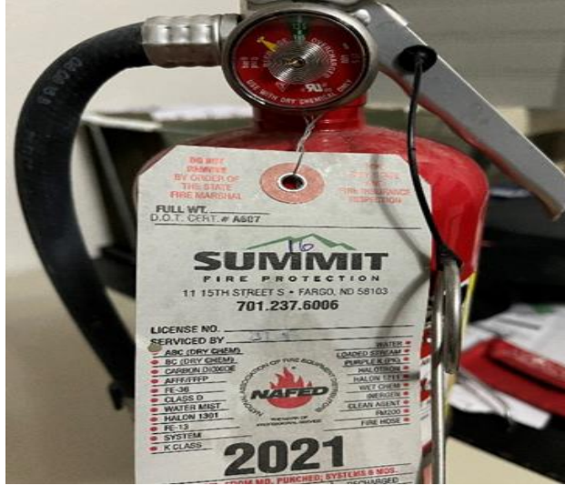
Photograph 2: Fire extinguisher not charged and outdated (last inspected 2021) (photo taken Nov. 18, 2024)
