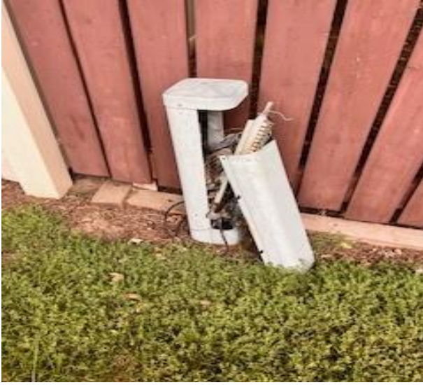
Photograph 5: Electrical box appears broken with exposed wires.
