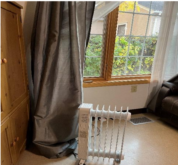
Photograph 13: Space heater placed near long drapes
