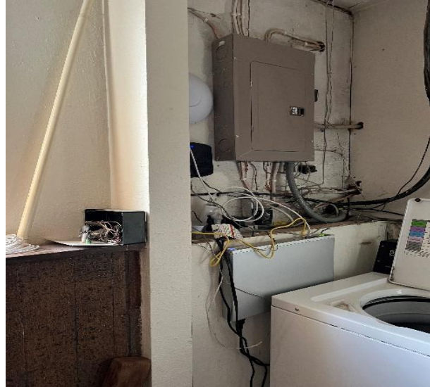
Photograph 6: Junction box with wires exposed
