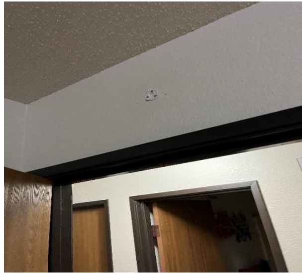
Photograph 18: Missing smoke detector on staff office wall, which was inoperable and found lying on staff desk
